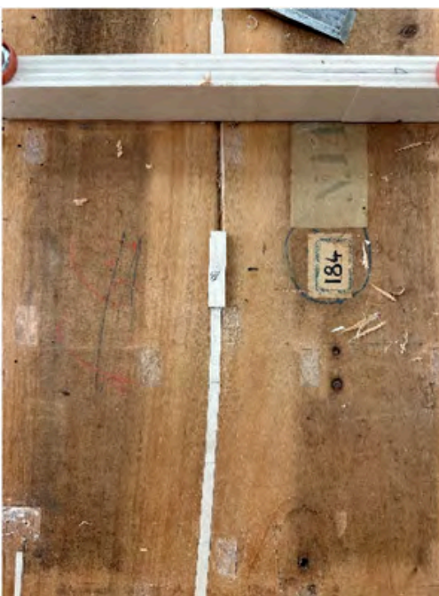
Replacement of previous restoration
